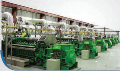
DG Power Plants
