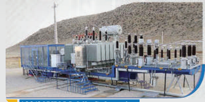
132/20KV Mobile Substation
