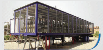
24KV Capacitor Banks
